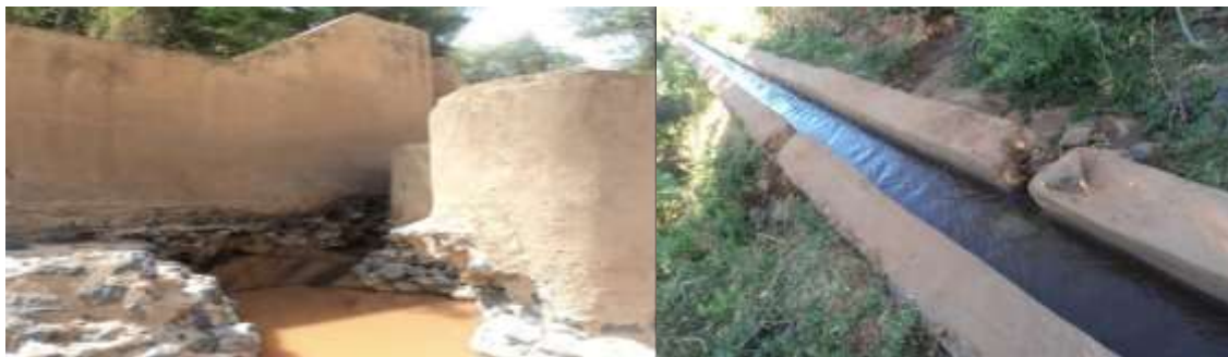
Figure 3. Mal-functioned hydraulic structures.
